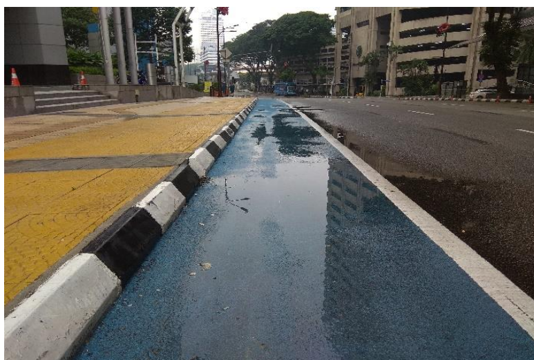
Figure 2: Water stagnant in a bicycle lane
