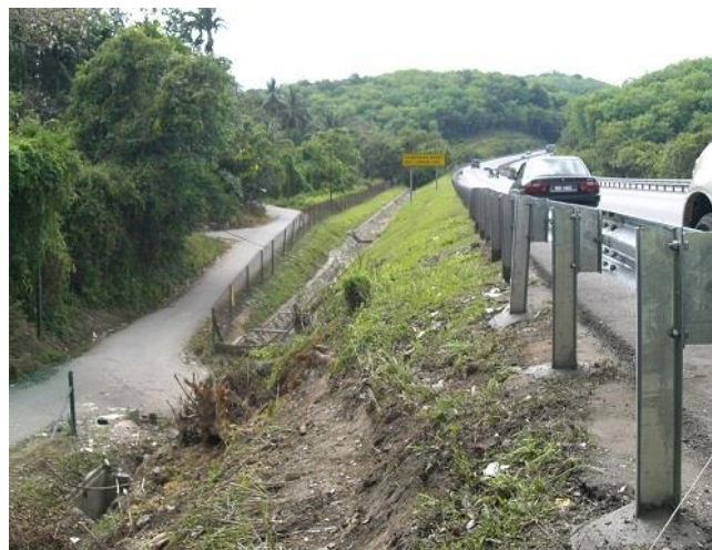
FIGURE 14: Inadequate dynamic deflection zone behind the guardrail
