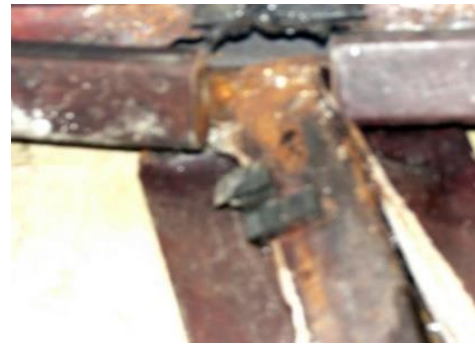
FIGURE 7: Rusted structure at the welded section
