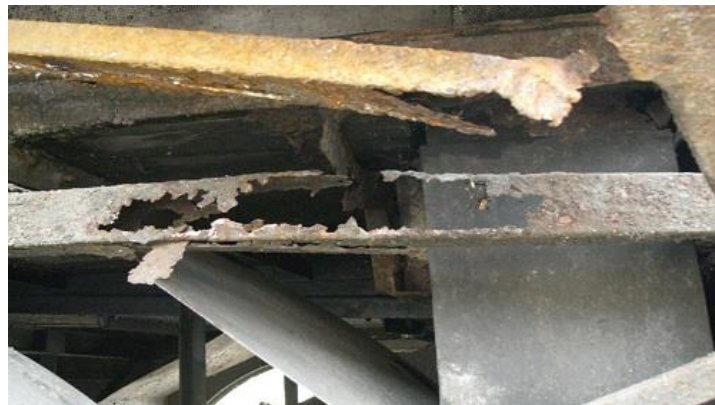
FIGURE 4: Severely rusted structures
